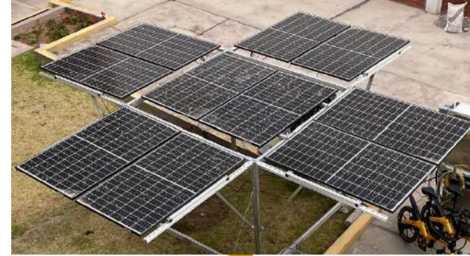
“Mariposa” Solar system
